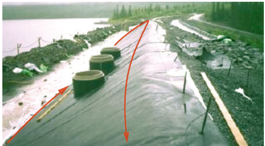
Installation of cable at Ajaure dam: the 1122m long cable was installed at two levels along the dam as a loop during construction.
