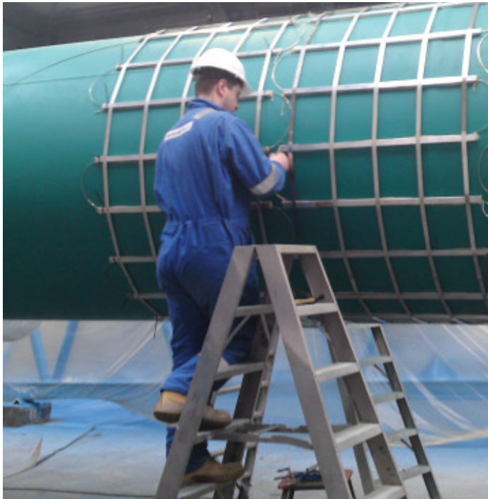
Sensornet engineer installing high temperature fibre in a mesh topology to provide complete coverage of Vessel 2
