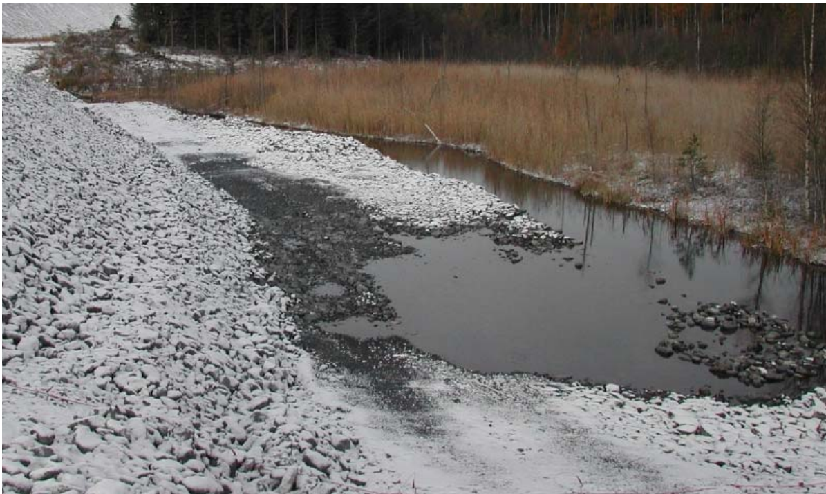
Figure 3 Seepage outflow area indicated by areas where the snow has melted.
