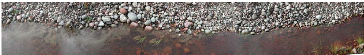
Figure 1 Concentrated outflow of muddy water and fines into a downstream ditch parallel to the dam.
