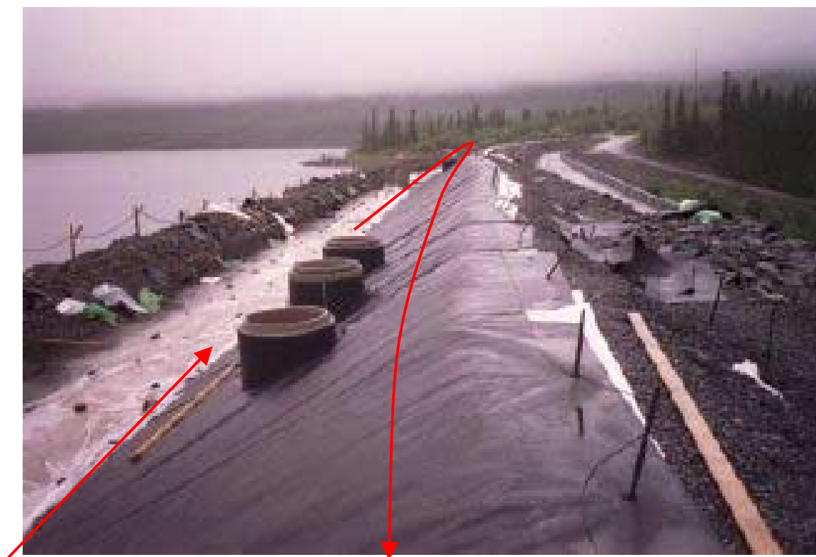
Figure 10 Location of the cables on the membrane. (The picture was taken during construction of the dam).
